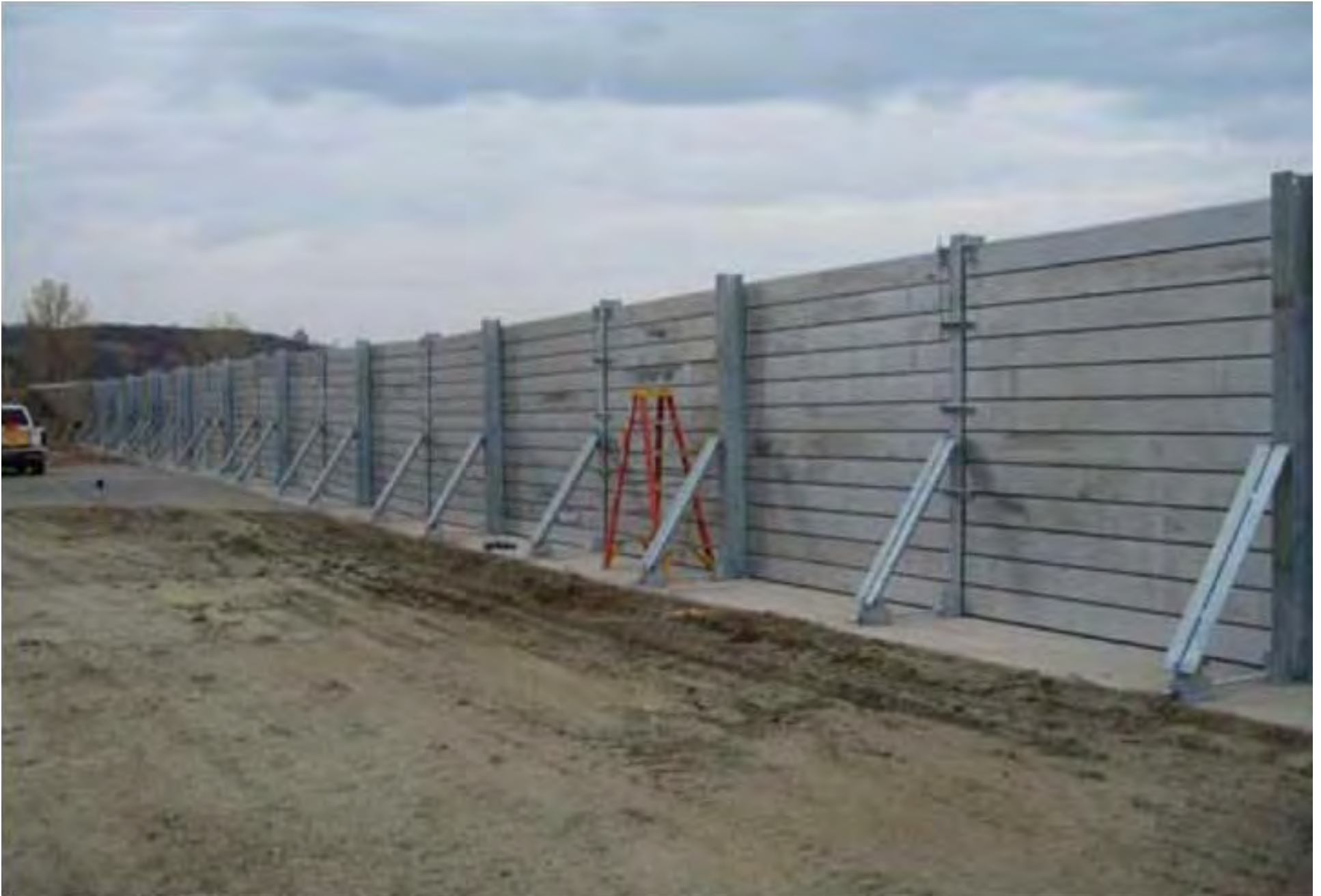
Temporary aluminum floodwall, upper Midwest, US.
